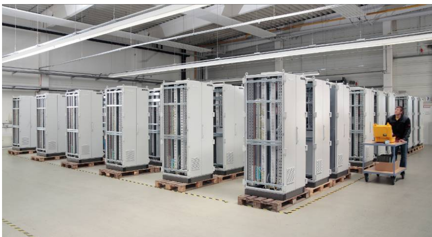
Fig. 4: A separate FAT facility allows an uninterrupted acceptance process, even for large numbers of units.
