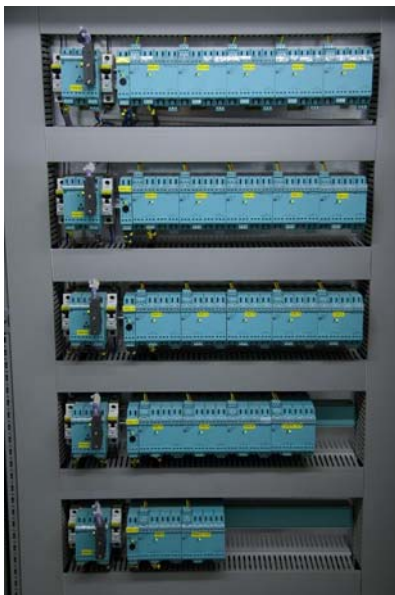
Fig. 3: A process control cabinet with the SK2 segment coupler is a model of tidiness and an efficient use of space. Up to Zone 1 field devices can be connected to each segment.
